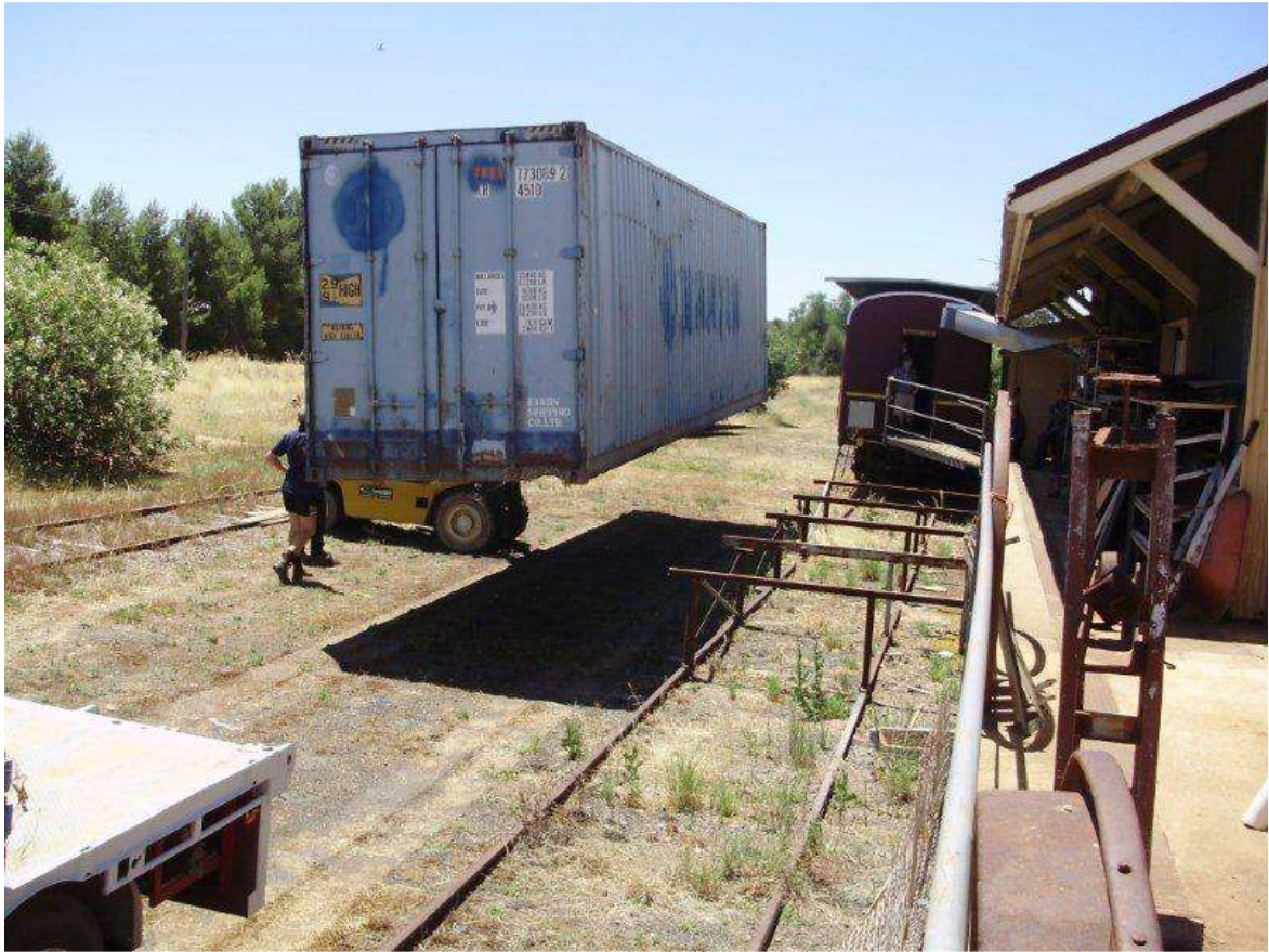
Placement of the Container making more room at the Grenfell Men's Shed.
